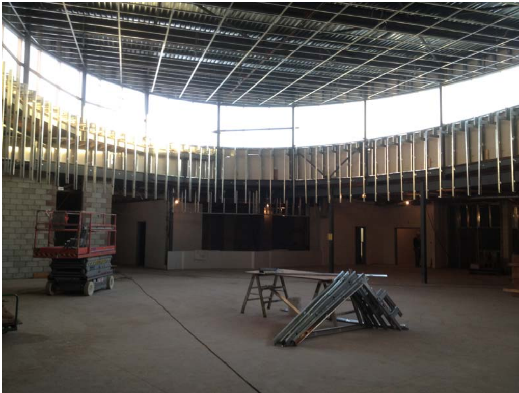
Common area - steel stud framing being put in place to accommodate drywall. Also a view of the front of the commercial kitchen
