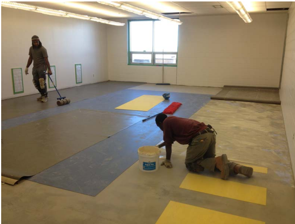
North classroom showing the installation of light fixtures and that flooring has commenced
