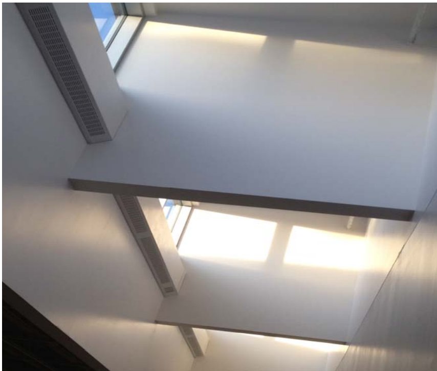
A look at a clerestory showing that the perimeter heating has been installed
