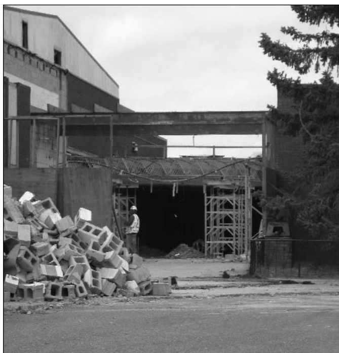
A new front entry shows construction continues inside and out at the modernization site.
