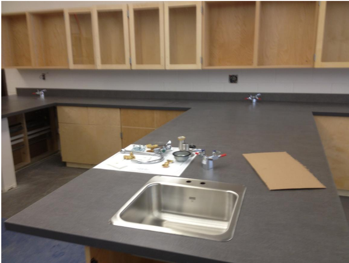
Science room mill work is in place and gas supply and sinks are being installed
