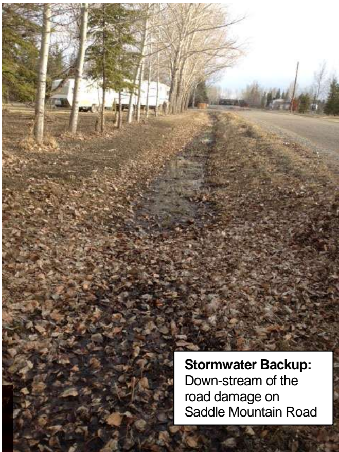
Blocked Culvert: Down-stream of the road damage on Saddle Mountain Road
