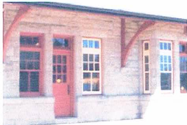
2. Detailed view showing primary window and original storm window in place, at right. 2012-07-05
