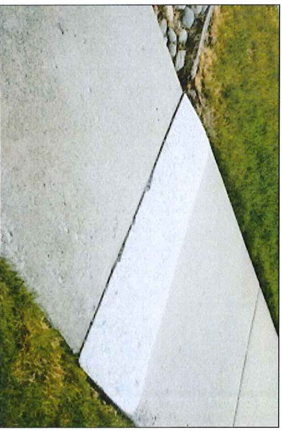
After Precision Concrete Cutting has completely and smoothly removed the trip hazard.
