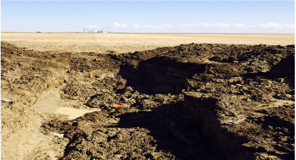
Photo of the dig location and new repair clamp installed by the Public Works
