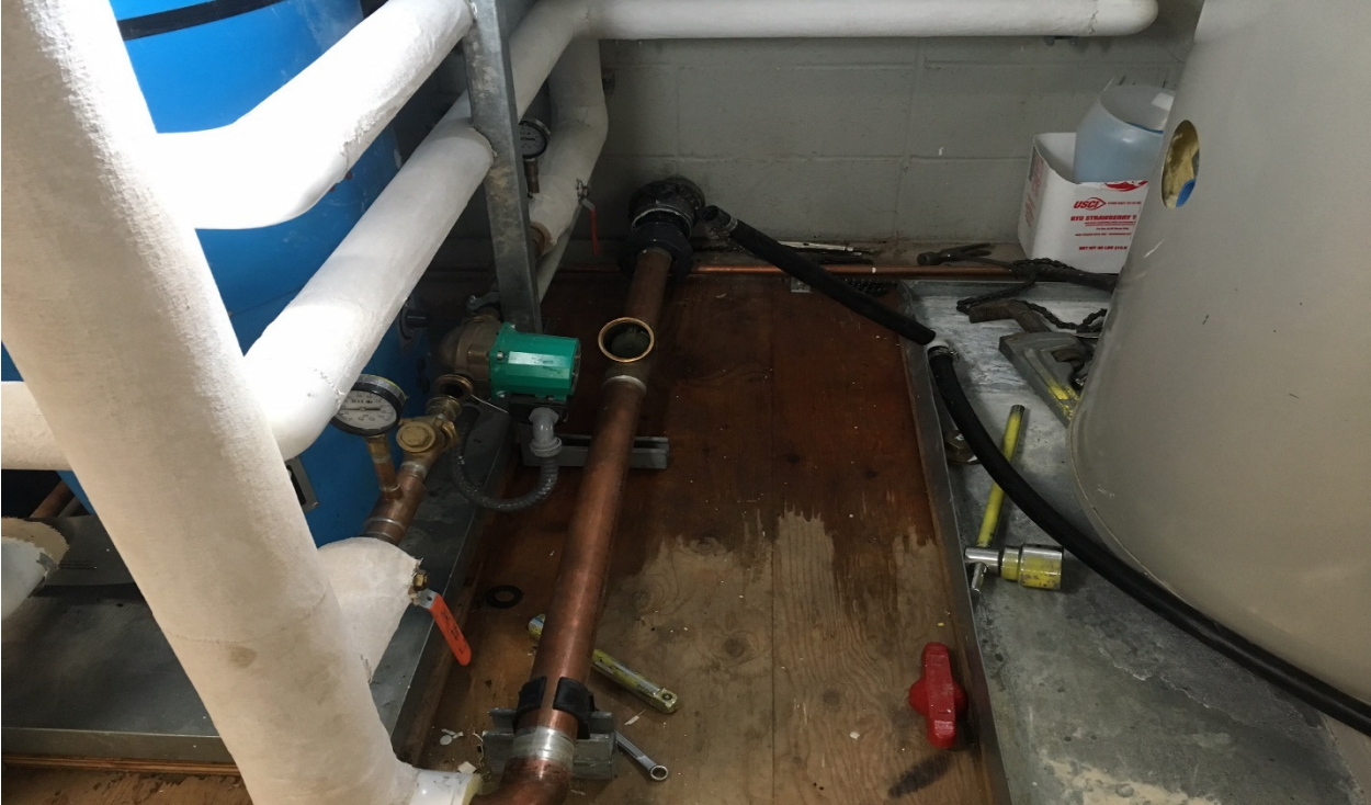
Back Check Valve check on DHW Supply above Maintenance Room Mezzanine (requires 2 new valves).
