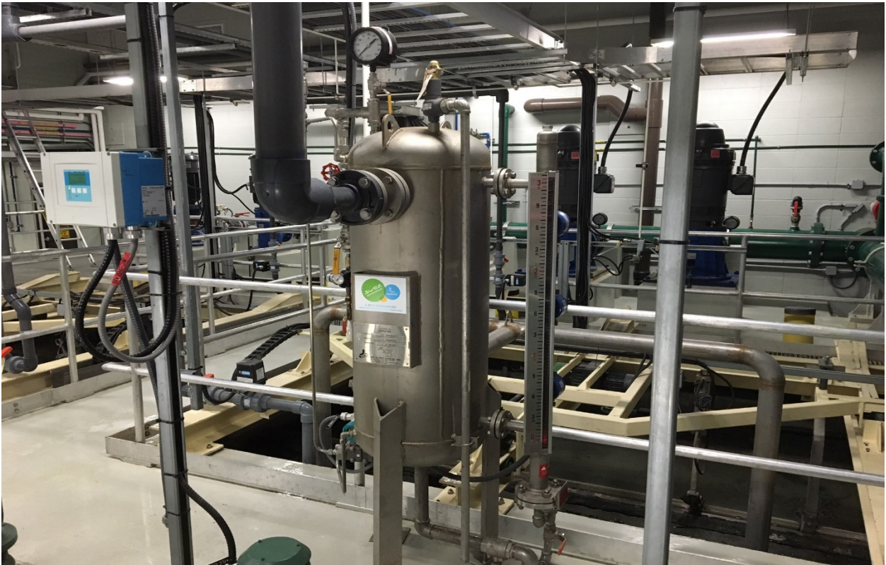
DAF #2 saturation tank vessel and controls
