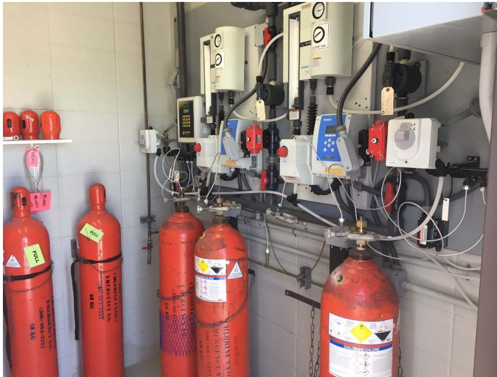
The Chlorine Room holds Twelve 68 kg Chlorine Gas Bottles.
